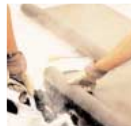
Bituminous membrane being applied to Hardrock Standard Roofing Board using pour and roll technique
