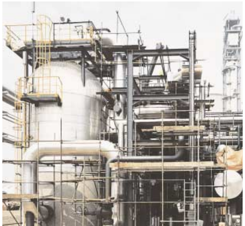
High temperature plant insulated using Rockwool Firebatt 825
