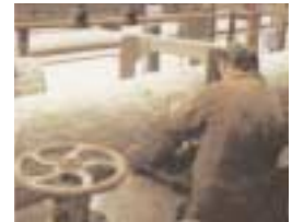
High temperature pipework
